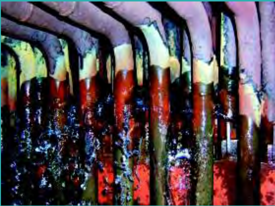
Boiler tube failure
